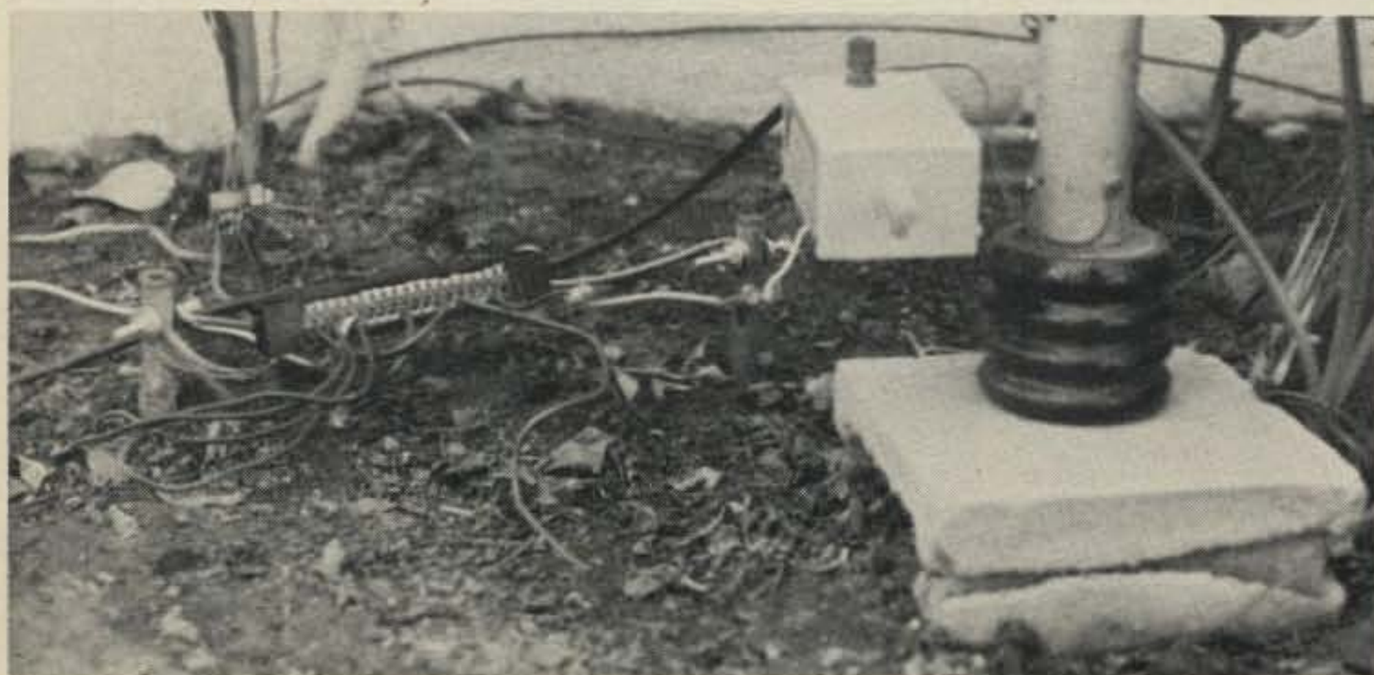
Photo of the antenna's base. See text for explanation.
